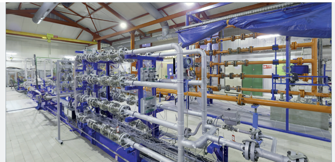
Hydrogen can now be supplied to the flowmeter test benches.
